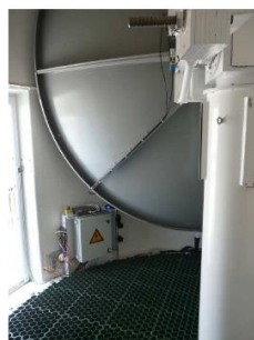
Surveillance and protection devices included
